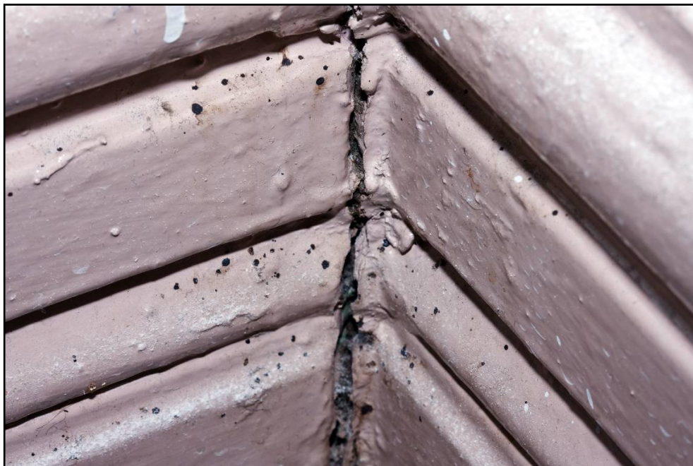
Figure 10. A large crack is present in the corner of the skirting and bed bug spotting is evident. Poor room integrity always makes bed bug control more challenging. ©2010 Department of Medical Entomology, Westmead Hospital, Westmead.
